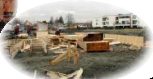
9 新堂地基工程正式展開 The preliminary construction of our new church has begun Dec 2001
