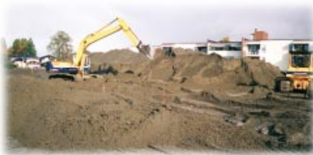
Preload sand is removed to make way for construction. 堆沙正被移走
